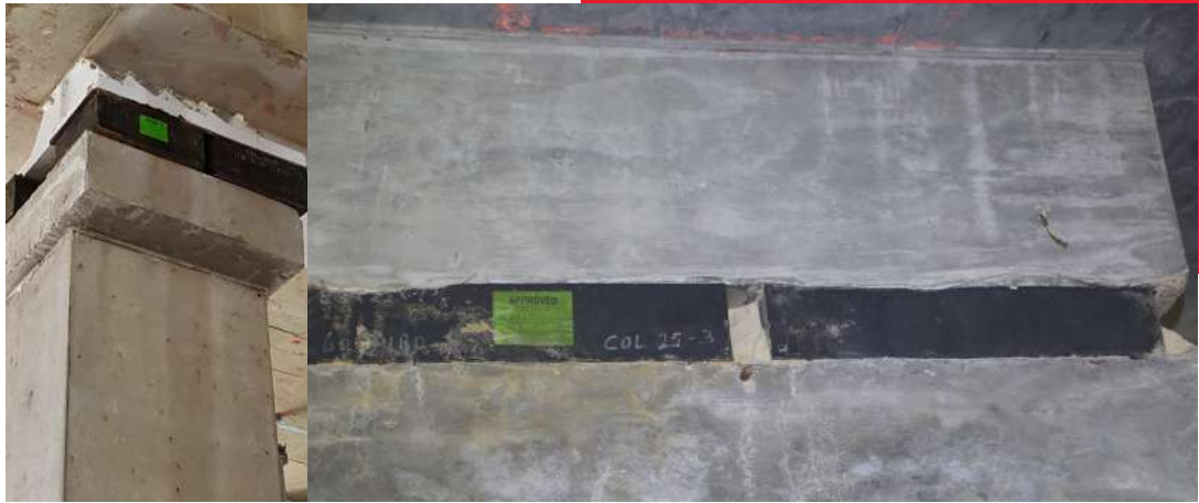
High load bearings at column capital with shear pins within bearing array
