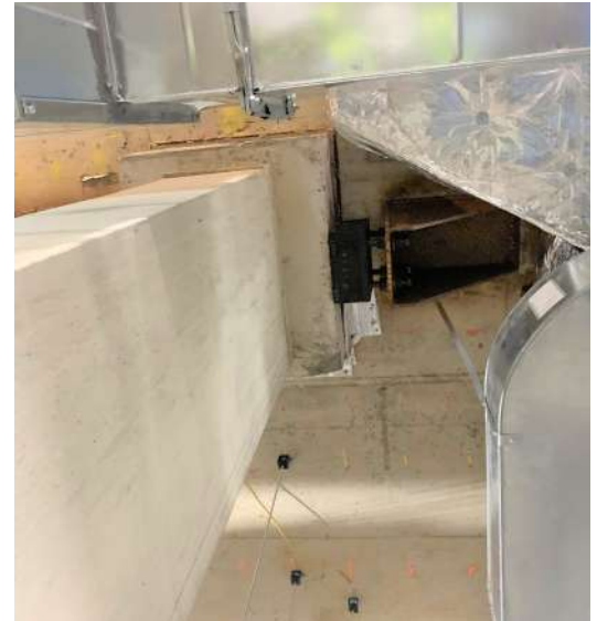
Lateral Restraint Blocks at walking columns
