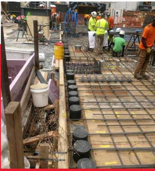
Shear key caps and bearings installed on top of shear wall. Sand packed to height of bearings
